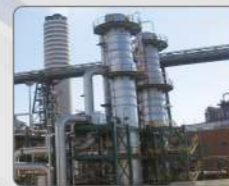
FLUE GAS DESULFURIZATION
