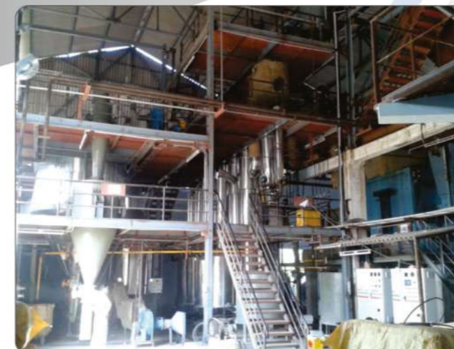
EVAPORATOR AND SPRAY DRYER
