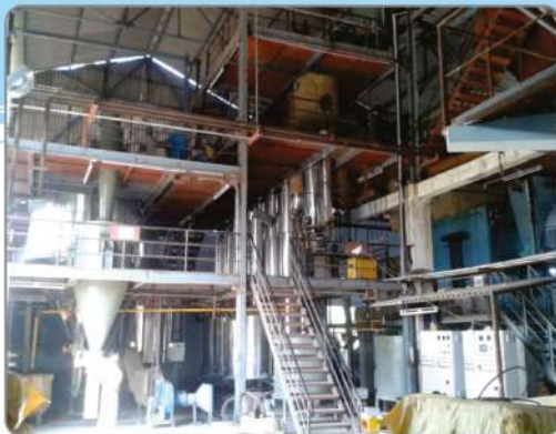
EVAPORATOR AND SPRAY DRYER
